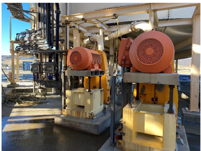
TAILINGS THICKENER PUMPS & MOTORS
