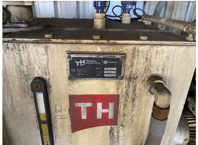
CONCENTRATION THICKENING AND FILTRATION
