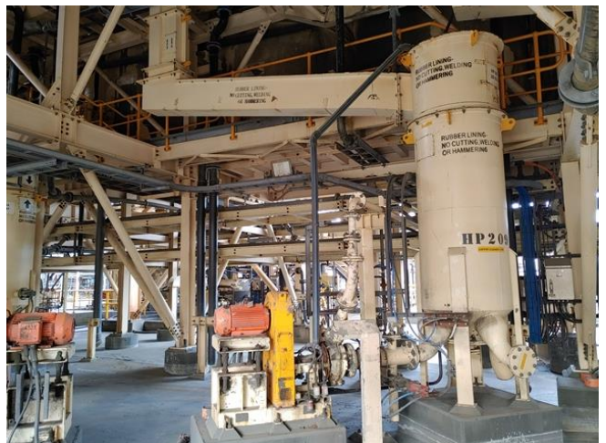
FLOTATION GROUND FLOOR TANKS AND PUMPS
