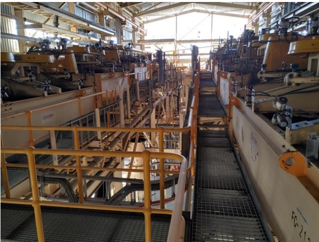
FLOTATION CELL OVERVIEW
