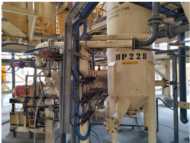
FLOTATION GROUND FLOOR TANKS AND PUMPS
