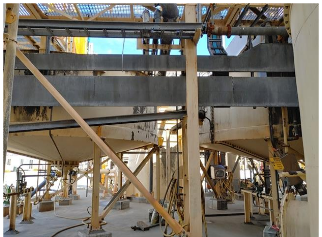
CONCENTRATION THICKENING AND FILTRATION
