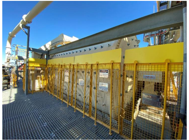
BALL MILL INFRASTRUCTURE
