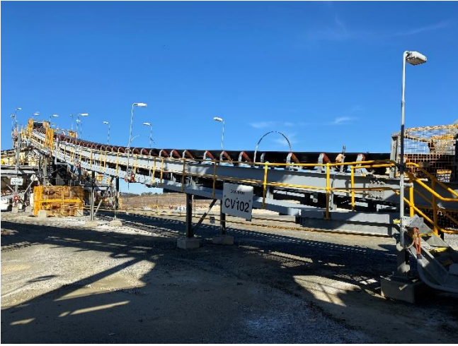
CONVEYOR CRUSHING AND SCREENING
