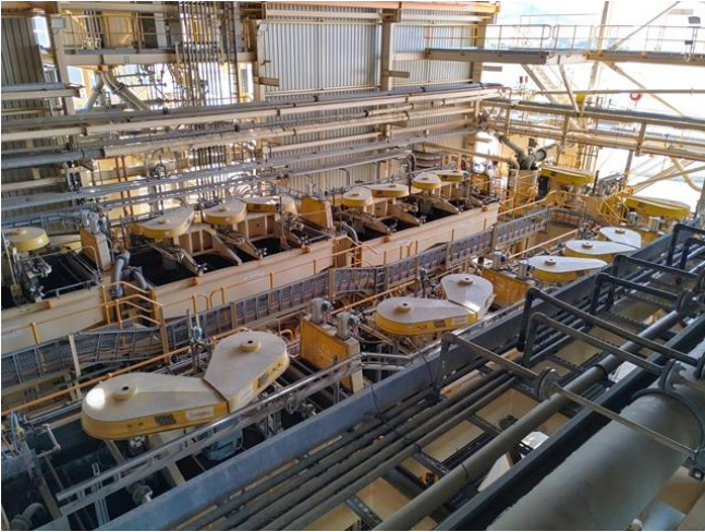
FLOTATION CELL OVERVIEW
