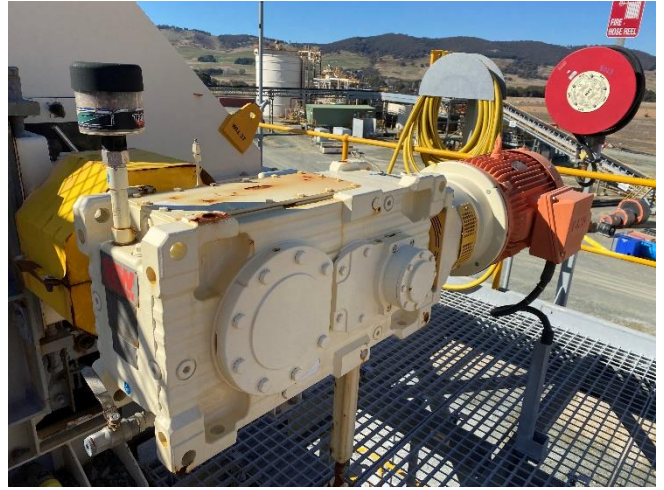
CRUSHING CIRCUIT MOTOR
