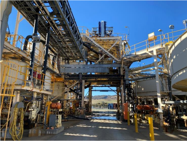
BALL MILL, ISAMILL AND TAILINGS THICKENER
