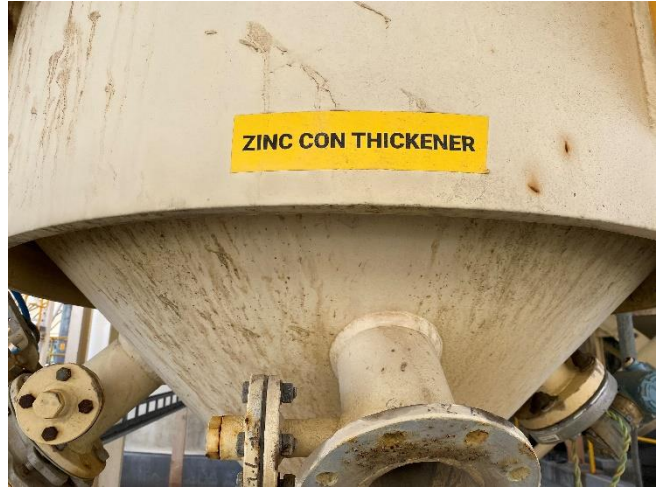
CONCENTRATION THICKENING AND FILTRATION
