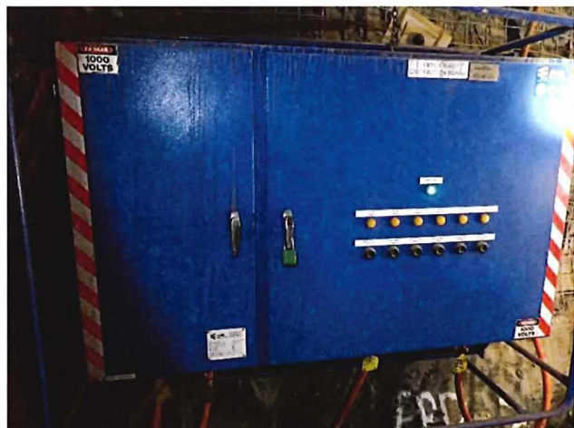
UNDERGROUND DISTRIBUTION BOARD
